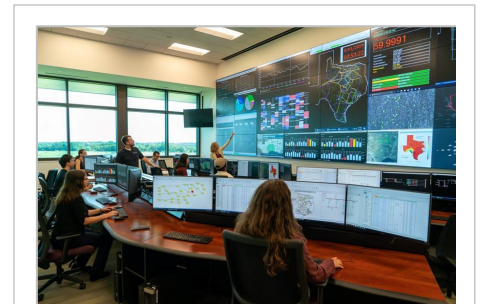
Smart Grid Control Room Lab is located at the Center for Infrastructure (CIR) building at the RELIS campus of Texas A&M University System.
